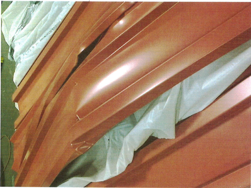
TYP. FAILED DISENGAGEMENT OF PANEL
