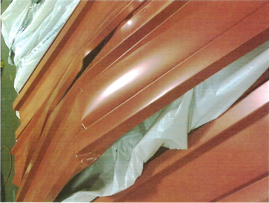
TYP. FAILED DISENGAGEMENT OF PANEL
